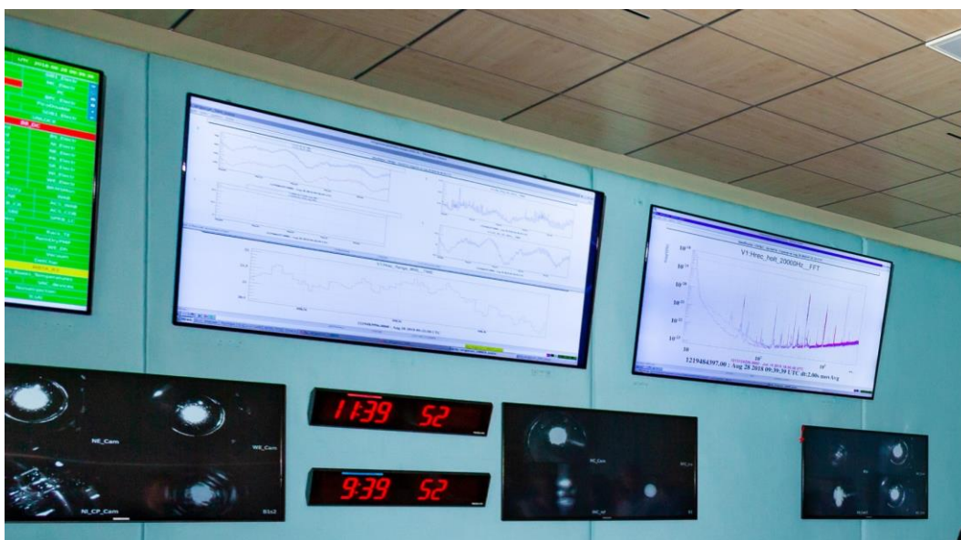
Figure 11 Virgo control room
