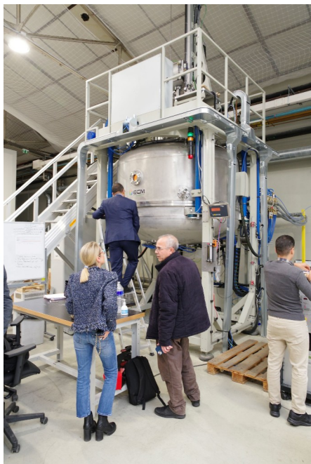
Inside and outside of the oven
